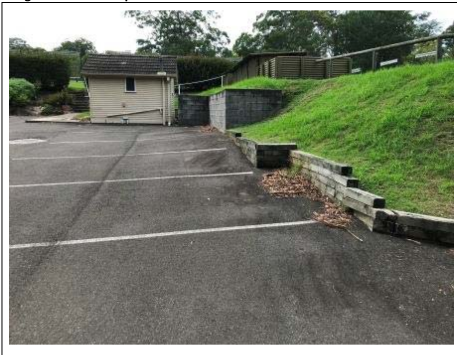
Image 6.6.1 View of potential fill embankment on north western corner of south western bowling green
