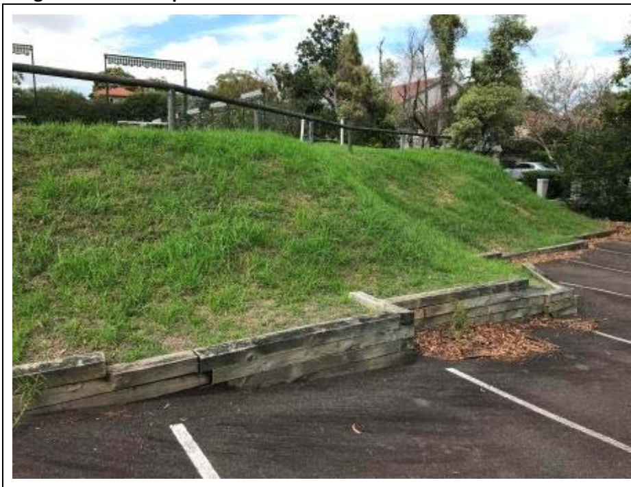
Image 6.6.2 View of potential fill embankment on north western corner of south western bowling green
