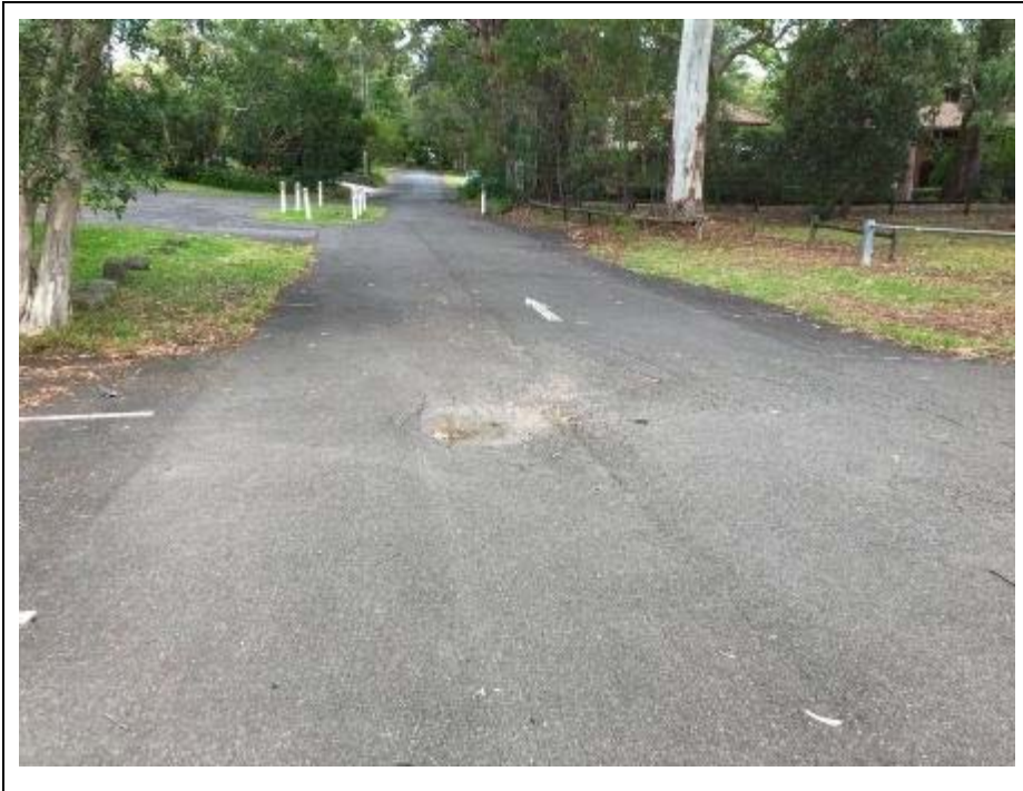
Image 6.2.2 View of a portion of the site access asphalt driveway in the western portion of the site, facing west
